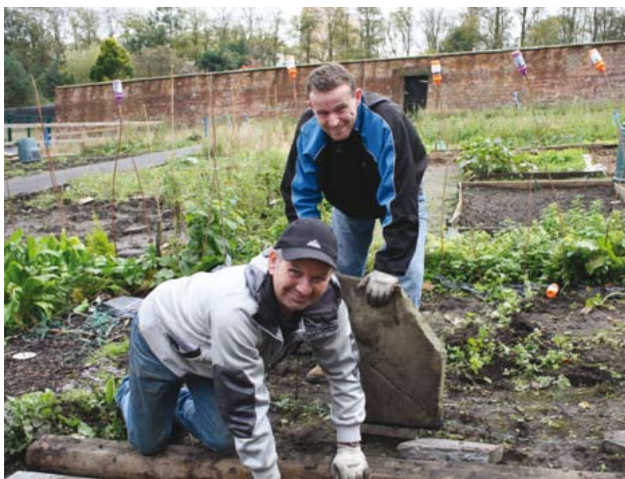
Pictured: Alex McLean (kneeling) and Peter Neely (standing) hard at work laying a new path at the allotment.
